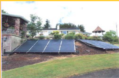
Eight 4x12 FAFCO SunSaver panels on GroundPro aluminum racks
